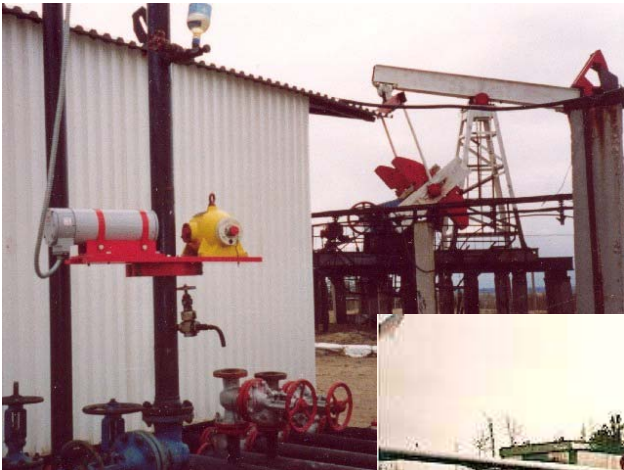
Single meter on beam-pump well
