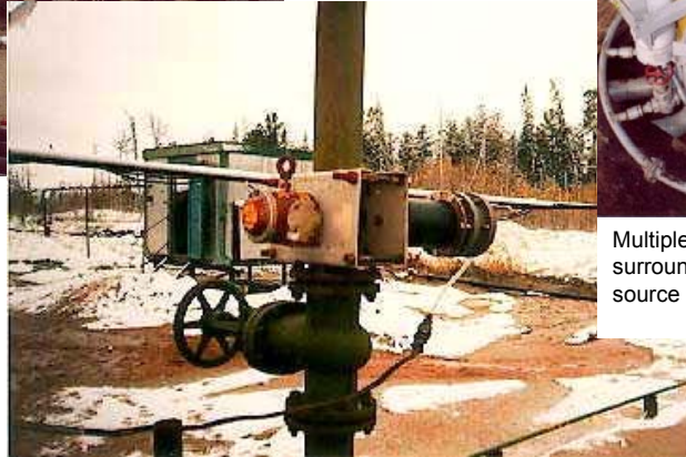
Prototype in field installation
