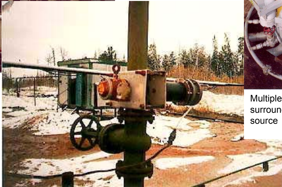
Prototype in field installation
