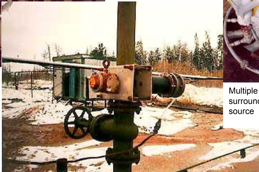
Prototype in field installation
